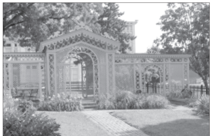
(above) The restored gazebo. (left) Dan and Rick Jente reconstruct the gazebo's central archway and lattice work.
